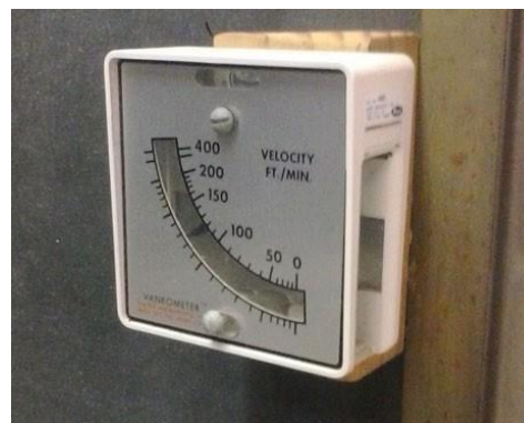
Figure 2. ECS hood Vaneometer. Note airflow reading above 100 LFM (arrow).
