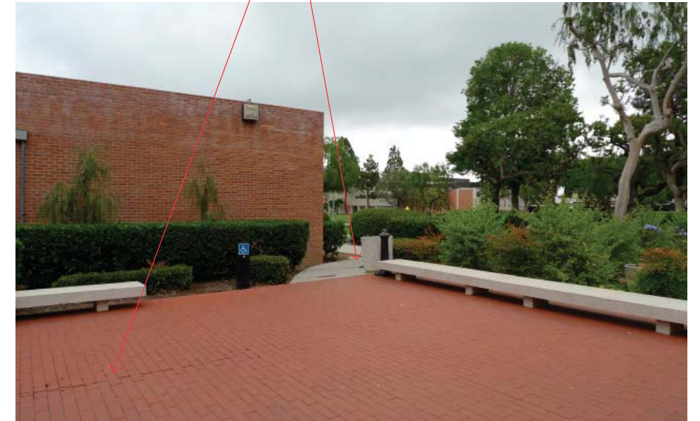
Bricks are buckling creating a safety hazard. Inadequate sidewalk.
