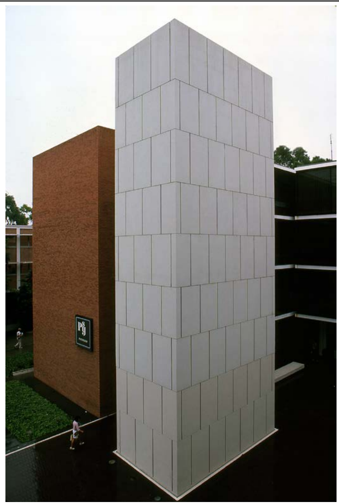
Image 10. Psychology Building, detail of vertical stair shaft, n.d. (CSULB Library Special Collections and University Archives)
