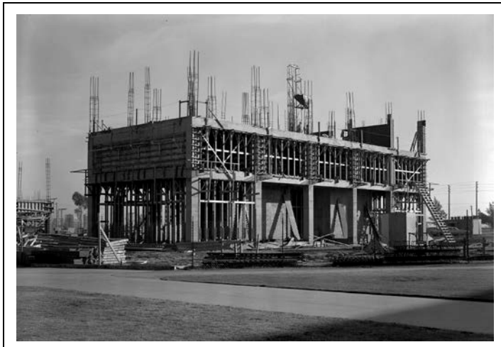
Image 6. McIntosh Humanities Building under construction, ca. 1966 (CSULB Library Special Collections and University Archives)
