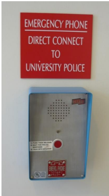
Building Hallways Wall Emergency Phone Boxes
