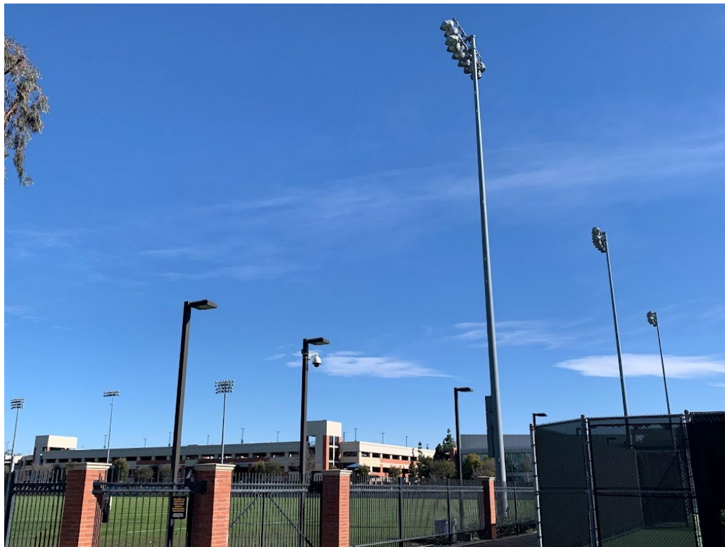
View 8 (North District): View from an interior pedestrian walkway looking east at the existing light poles at George Allen Soccer Field.
