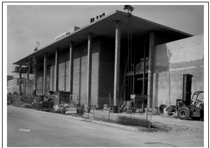
Image 7. Theatre Arts Building under construction, 1971 (CSULB Library Special Collections and University Archives)
