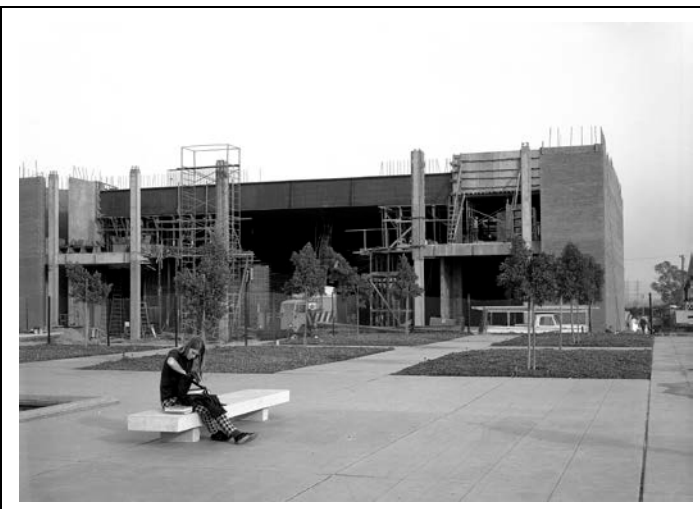
Image 6. Theatre Arts Building under construction, 1971 (CSULB Library Special Collections and University Archives)
